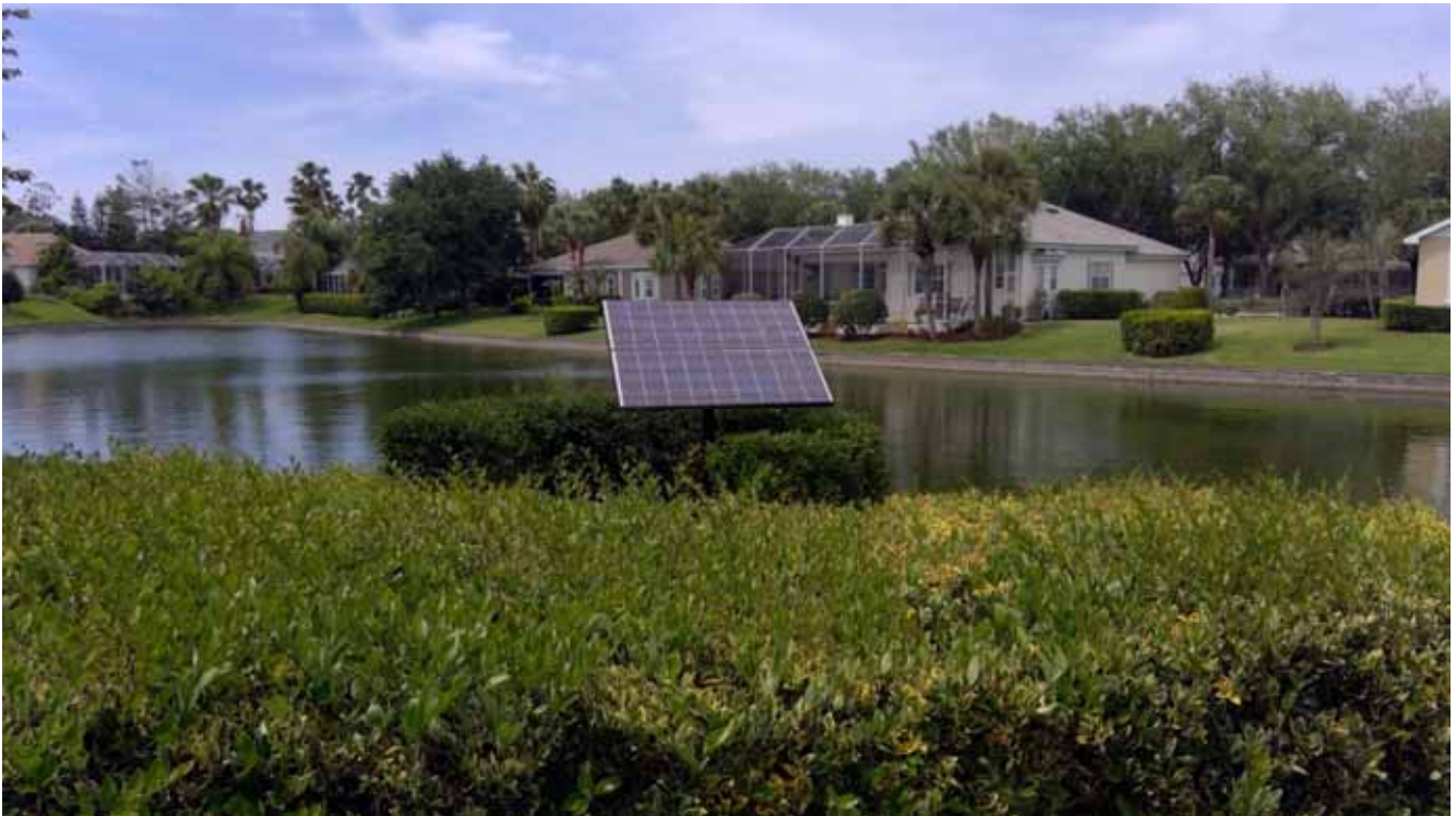
Solar Panel - Lake Aerator
