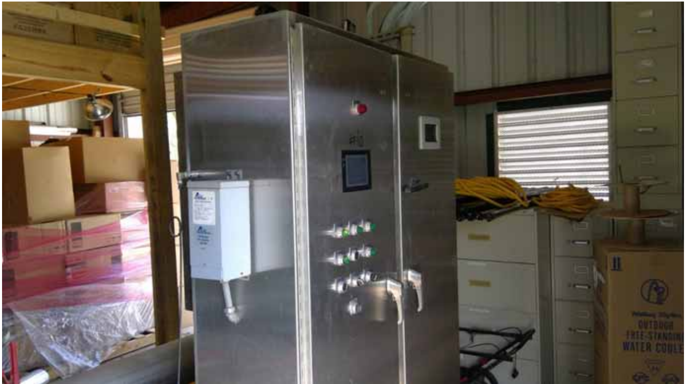
Irrigation Control Panel
