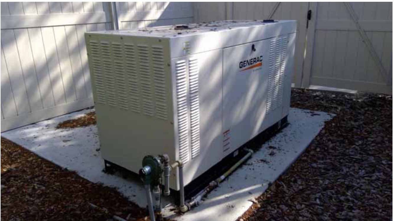
Generator - Clubhouse VC
