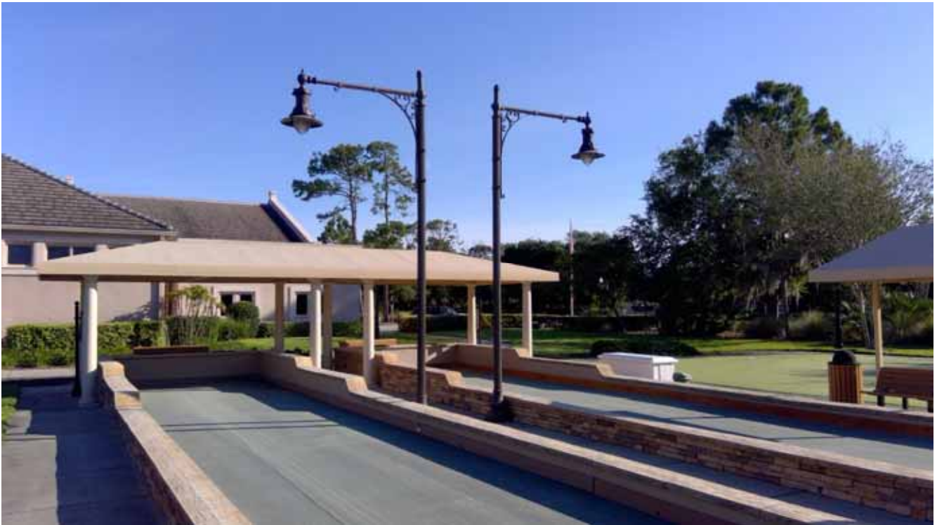
Lighting - Bocce Ball Ct VC
