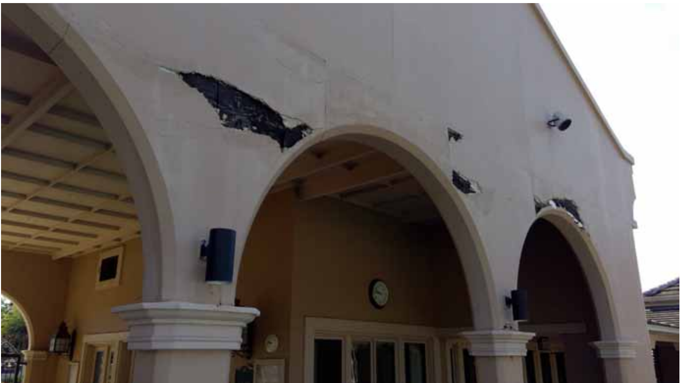
Stucco Delamination - VC
