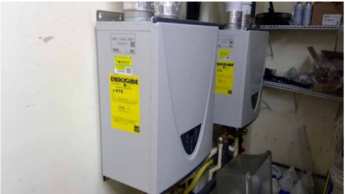
Water Heaters - Clubhouse VC
