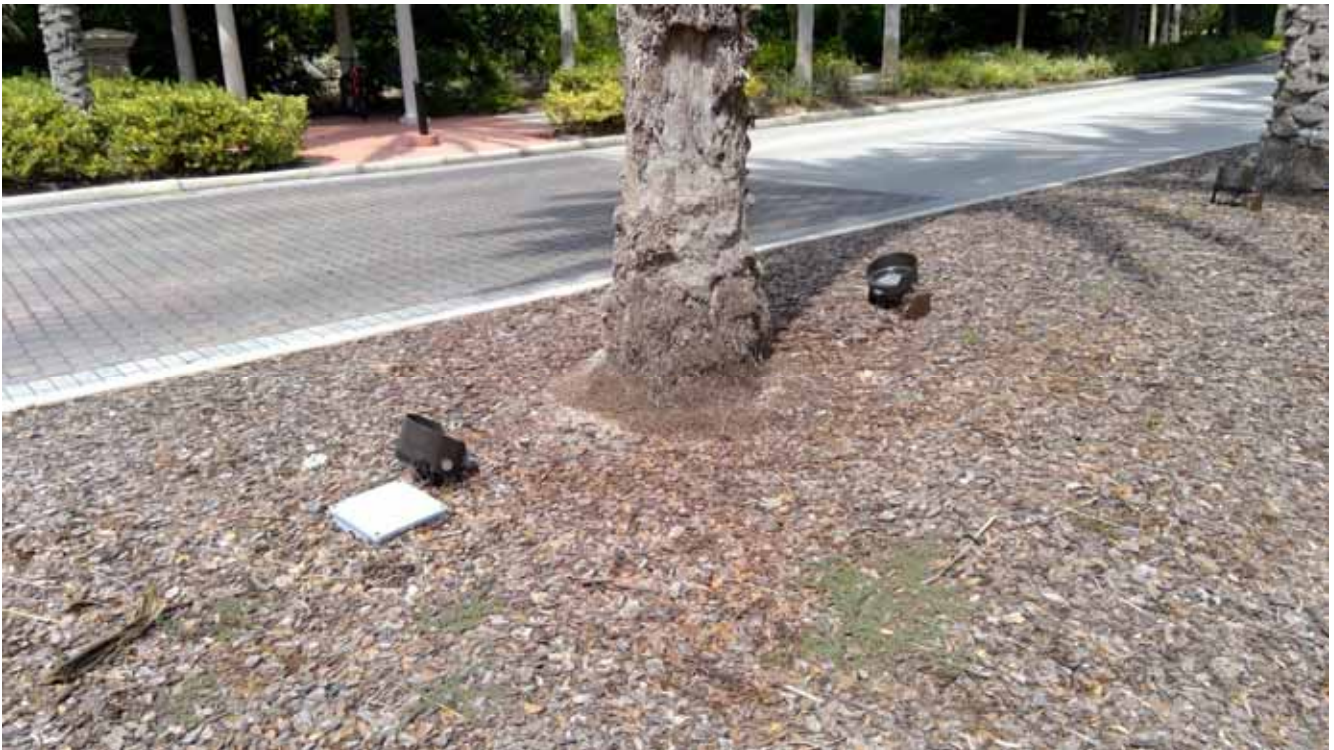
Entry Lighting - South
