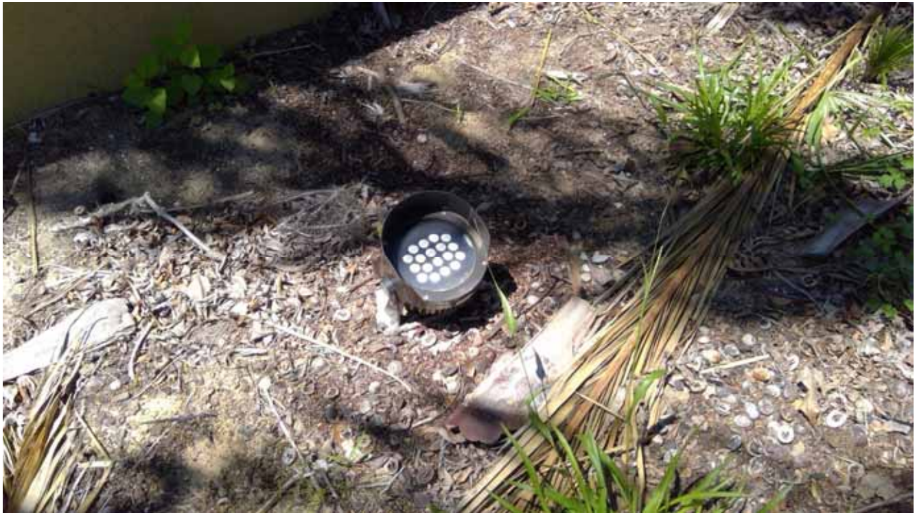
Entry Lighting - North
